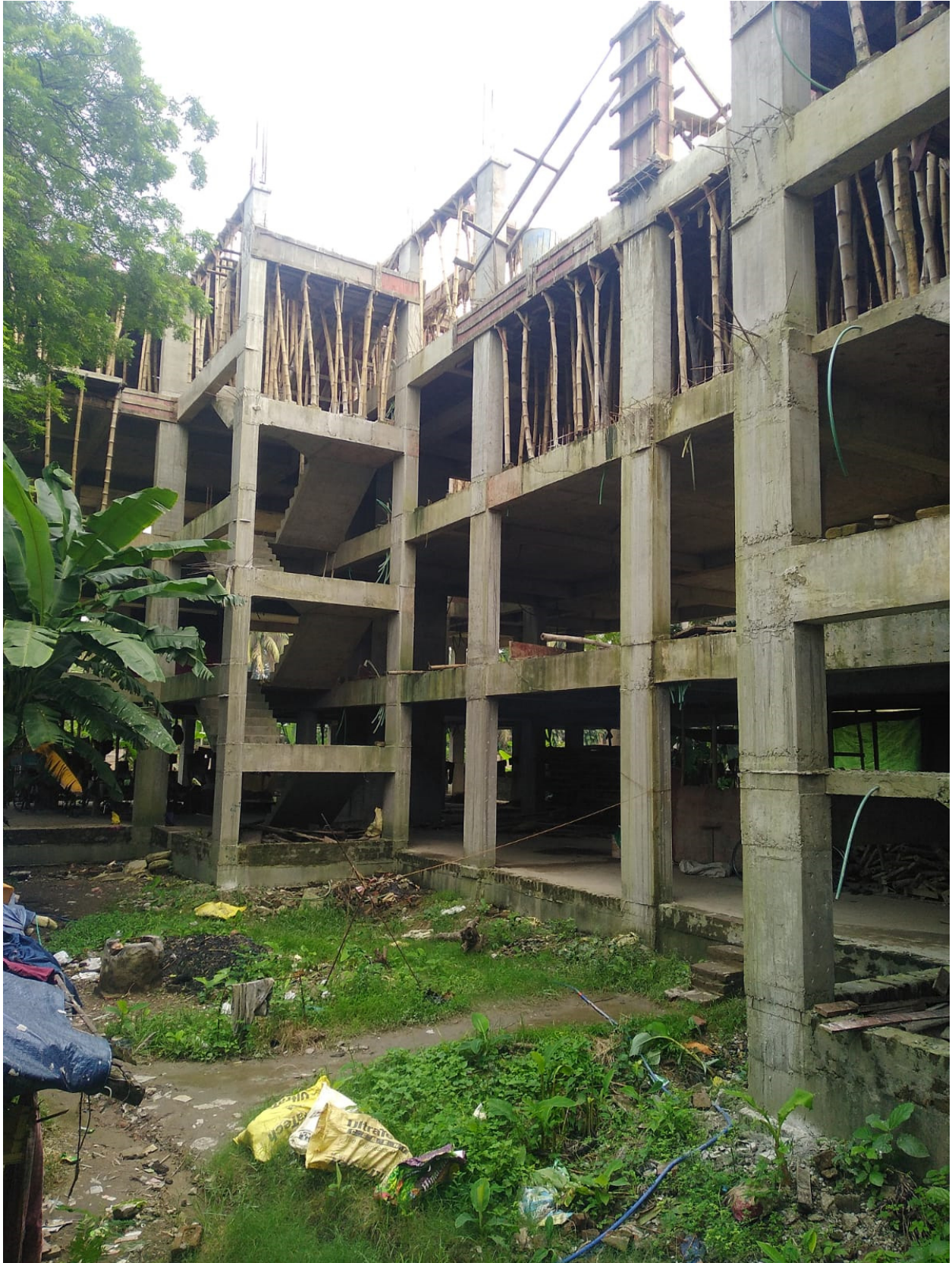
GLOBAL RESIDENCY_1 st & 2 nd FLOOR ROOF CASTING COMPLETED AND 3 rd FLOOR ROOF CASTING WORK UNDER PROGRESS
